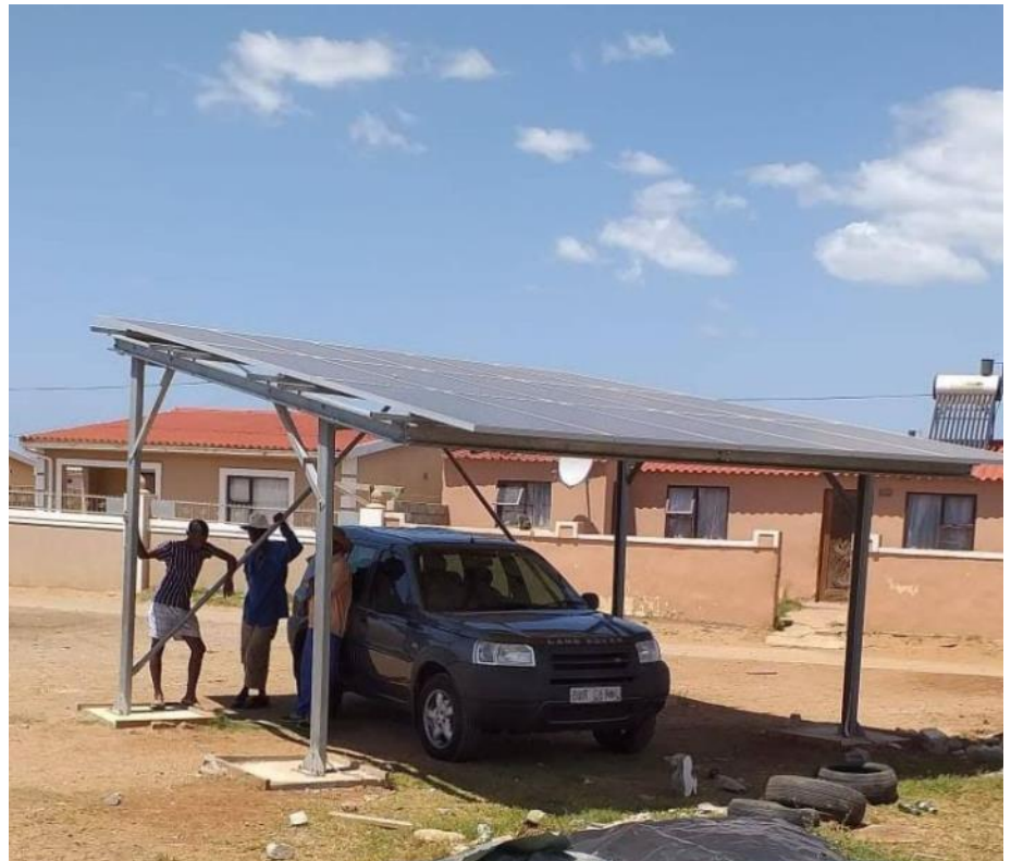
The carport with 15 PV panels that generated 5kw of electricity that was fed straight into the municipal grid
